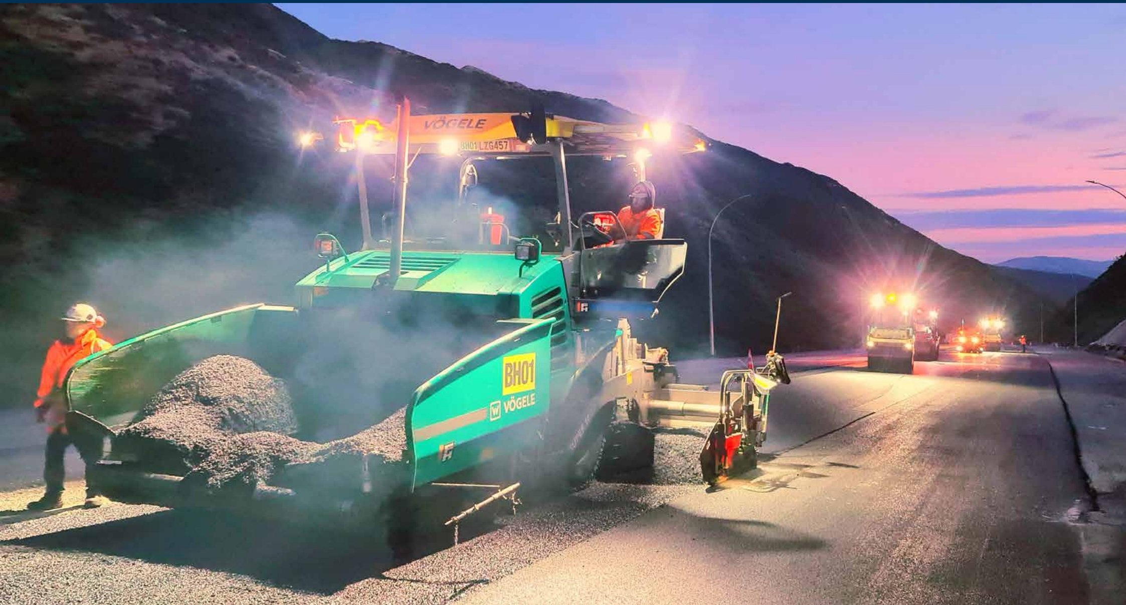
Paving the new Transmission Gully highway Photo by Caleb Clark, Fulton Hogan
