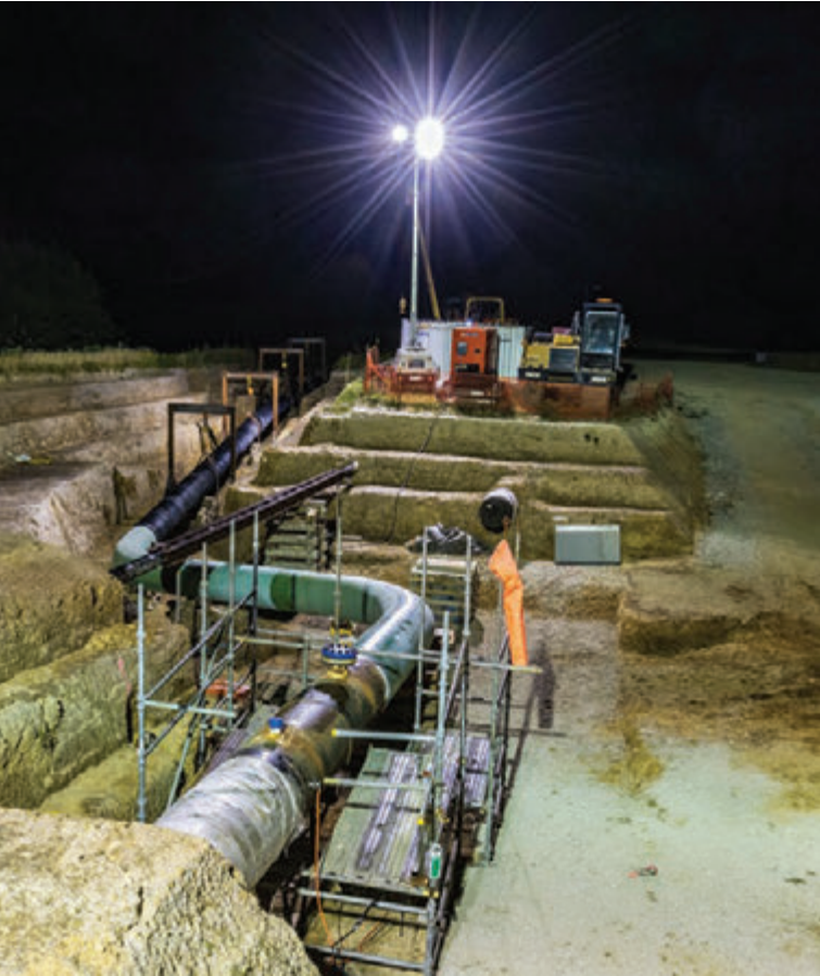
Maui Gas Pipeline – First Gas
