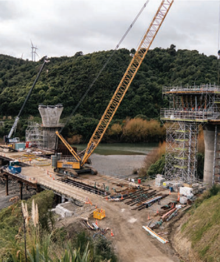
Work on the three concrete piers for the 300 metre long Parahaki Bridge over the Manawatū River
