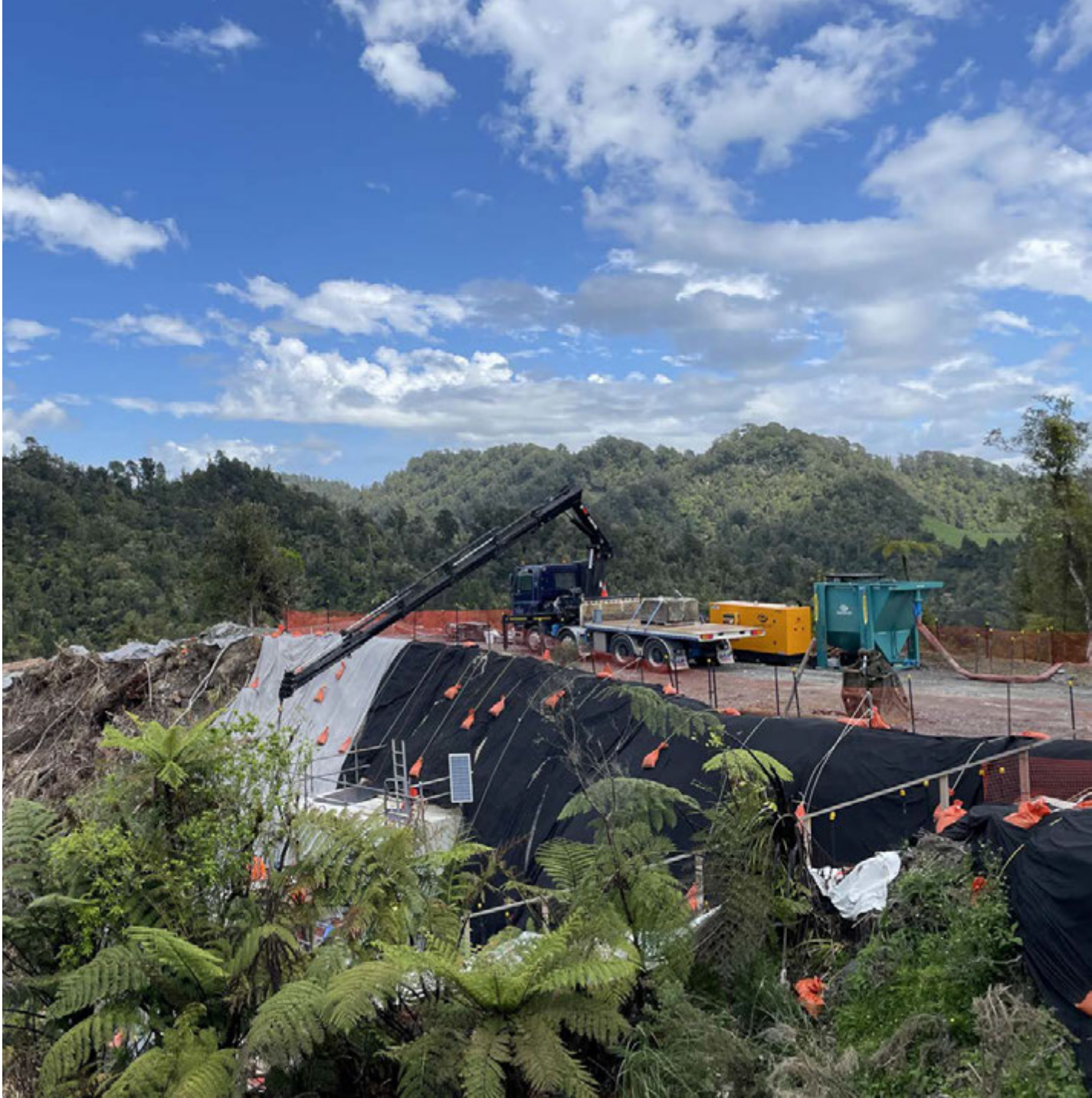
Mount Messenger Bypass tower site, looking towards the south anchors just before the installation of the tower
