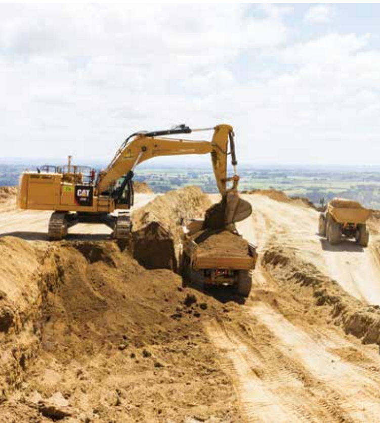
Excavation works on the new Manawatu-Tararua highway – Te Ahu A Turanga Alliance
