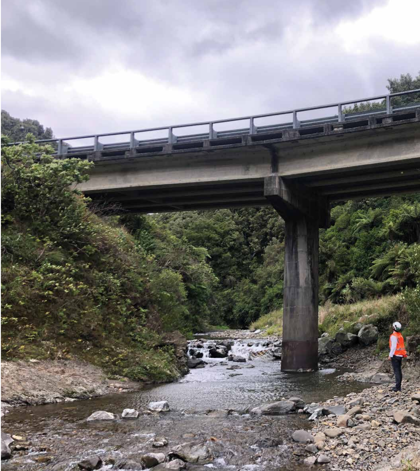
Applying new methodologies resulted in an excellent outcome for bridge strengthening in the Bay of Plenty.
