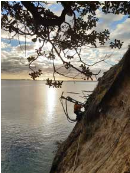
Paul from Groundfix, Auckland took this epic photo of Mathieu, a Groundfix rope access technician drilling soil nails for cliff stabilisation.
