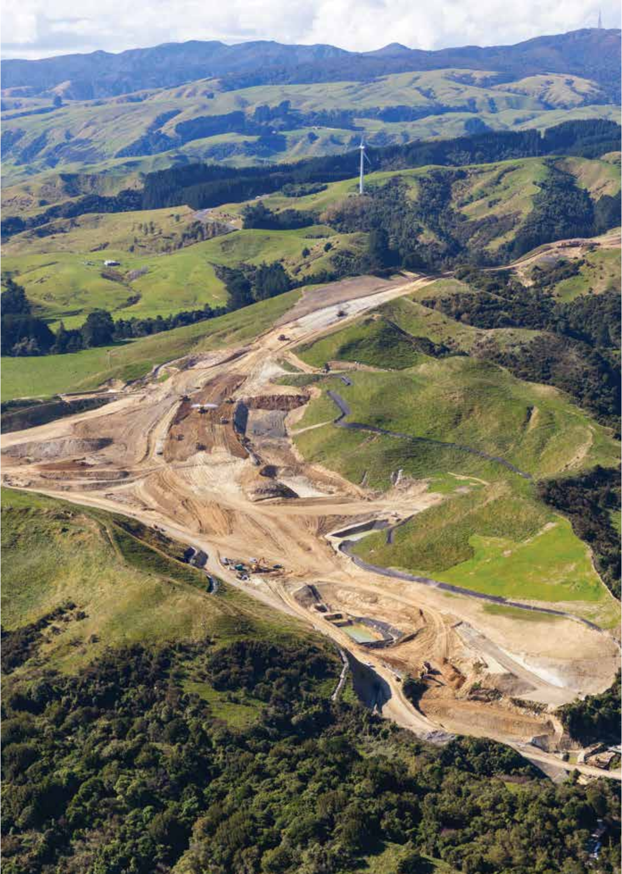
Earthworks for the new Te Ahu a Turanga Manawatu Tararua Highway in progress – Te Ahu a Turanga Alliance.
