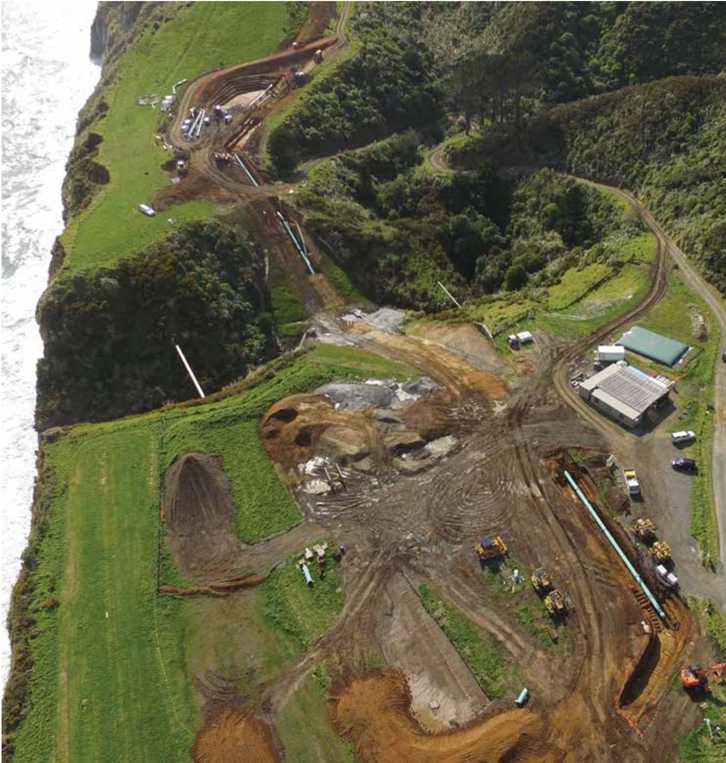
The replacement of a section of the Maui gas pipeline on the west coast.
