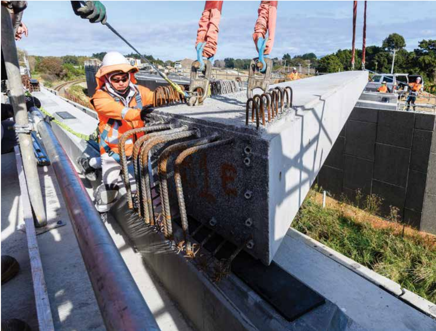
Fixing a concrete bridge beam into position at Mary Crest Bridge, Peka Peka to north of Otaki section of the Kapiti Expressway.
