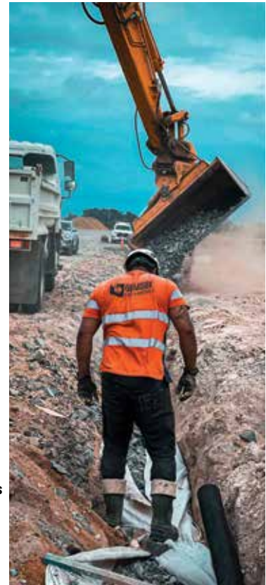
Cairo from Ormsby Civil Construction, Hamilton took this shot of an Ormsby Civil Construction field worker putting in the hard yards in the Waikato region.
