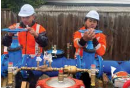
Ben from Dempsey Wood, at Wellington – a great chance to immerse the team to a few new aspects of Watermain Installation.
