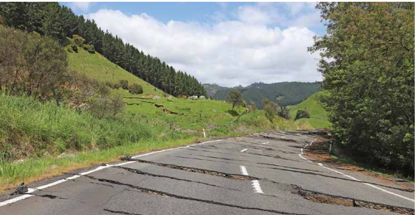
Whanganui - Raetihi SH4 road rippling.
