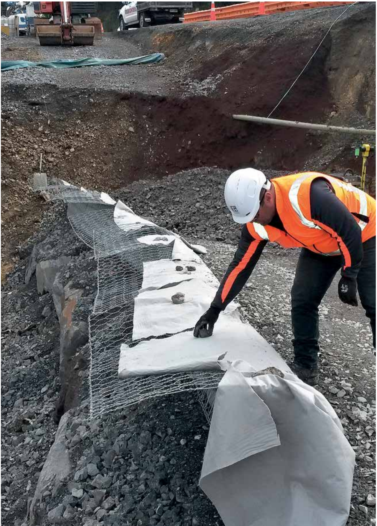
Installing the first layer of terramesh on a 6m deep rock spall base; Hautapu slip repairs, Northland 2017.
