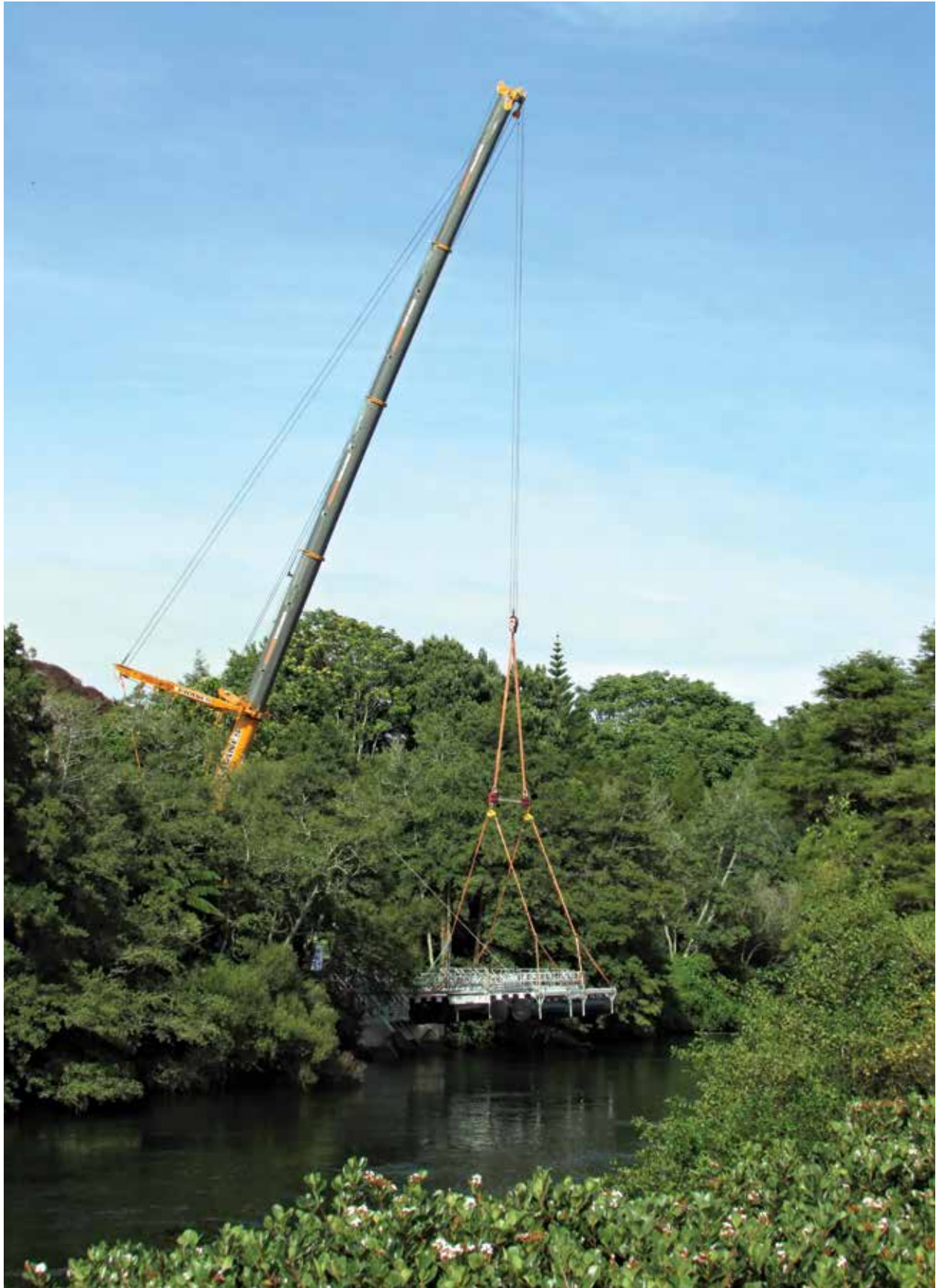
A Hamilton water treatment plant being craned into place on the Waikato River.
