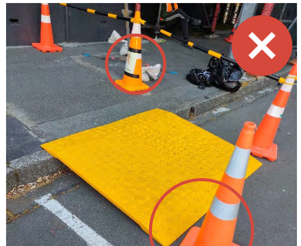
The use of paper taped to a cone has meant the sign has deteriorated and hardly visible. The cone makes the ramp narrower which is particularly problematic for people using a wheelchair. Image Credit Iv: Betty Mitrova.
