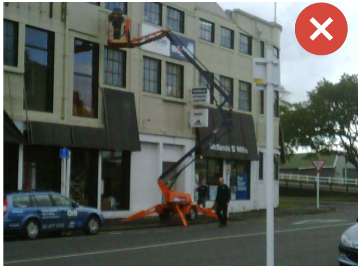
The person working on the elevated work platform has tools and materials that may fall onto the walkway below. The EWP is blocking the footpath. Image Credit xxx: Peter Graham.
