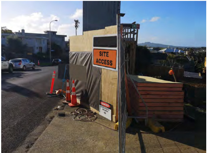
Site access and exit in this location would be very challenging. Pedestrians interacting in the same place as entering vehicles and a blind corner of hoarding close to a live traffic lane. This location would require a number of control measures to ensure the safety of site entry and exit activity. Image Credit lxiii: Parallax.
