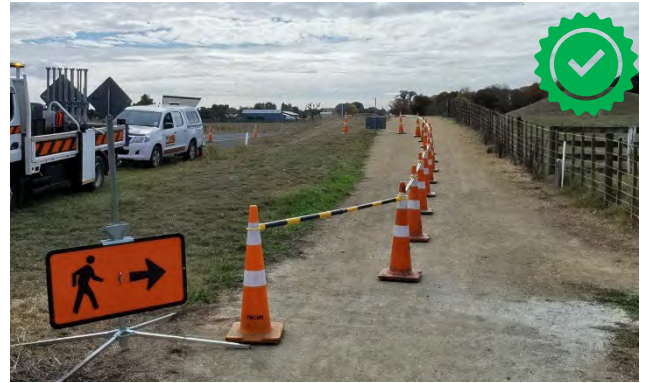
This example shows a narrowed existing path with a method to prevent access to the hazard area and directional signage. One improvement would be ensuring the method preventing access is particularly clear at the entry points (closest to the camera) to make sure pedestrians can't get through, especially at the point of the change in their direction. Image Credit xliii: Traffic Management Hawkes Bay.
