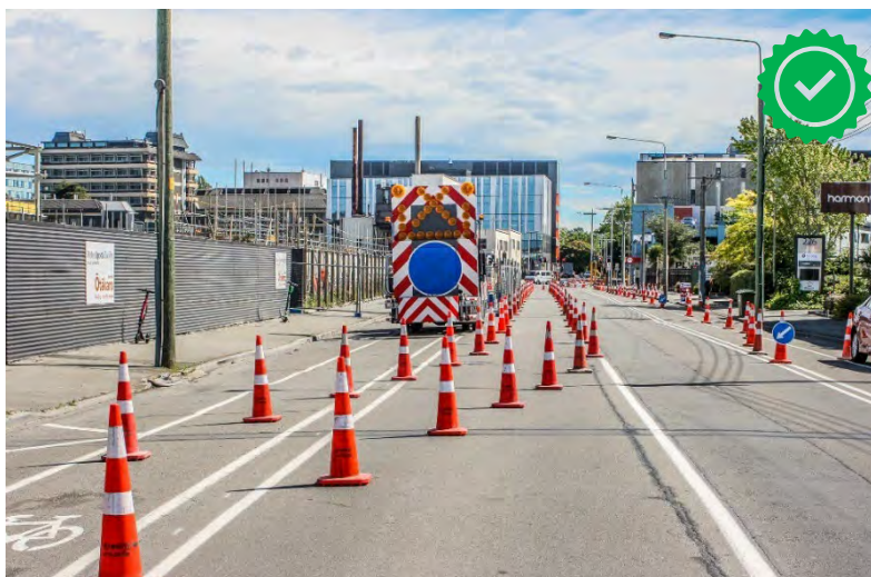
This example shows a clear and well aligned temporary cycle lane diversion. One improvement would be adding a method to prevent cyclists riding through the cones (especially at the diversion location). Image Credit xlvi: Whites Traffic Management.
