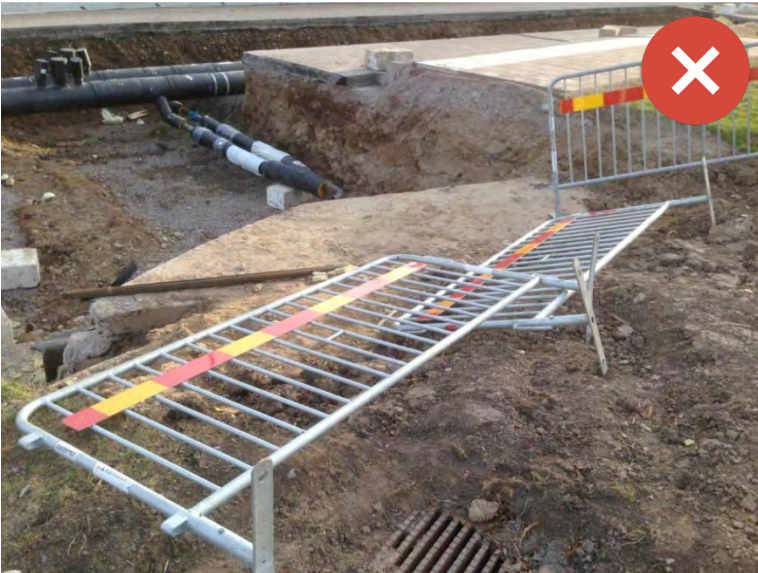
Fences to prevent access to hazards but have fallen over, creating risk for vulnerable road users. Image Credit Ivi: Sweden National Road and Transport Research Institute 441 .
