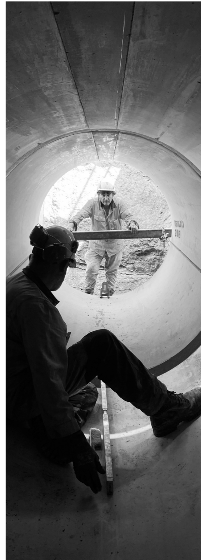
Michelle from E.N Ramsbottom Ltd, at Porirua, Wellington - Installation of a new 1500dia stormwater pipe
