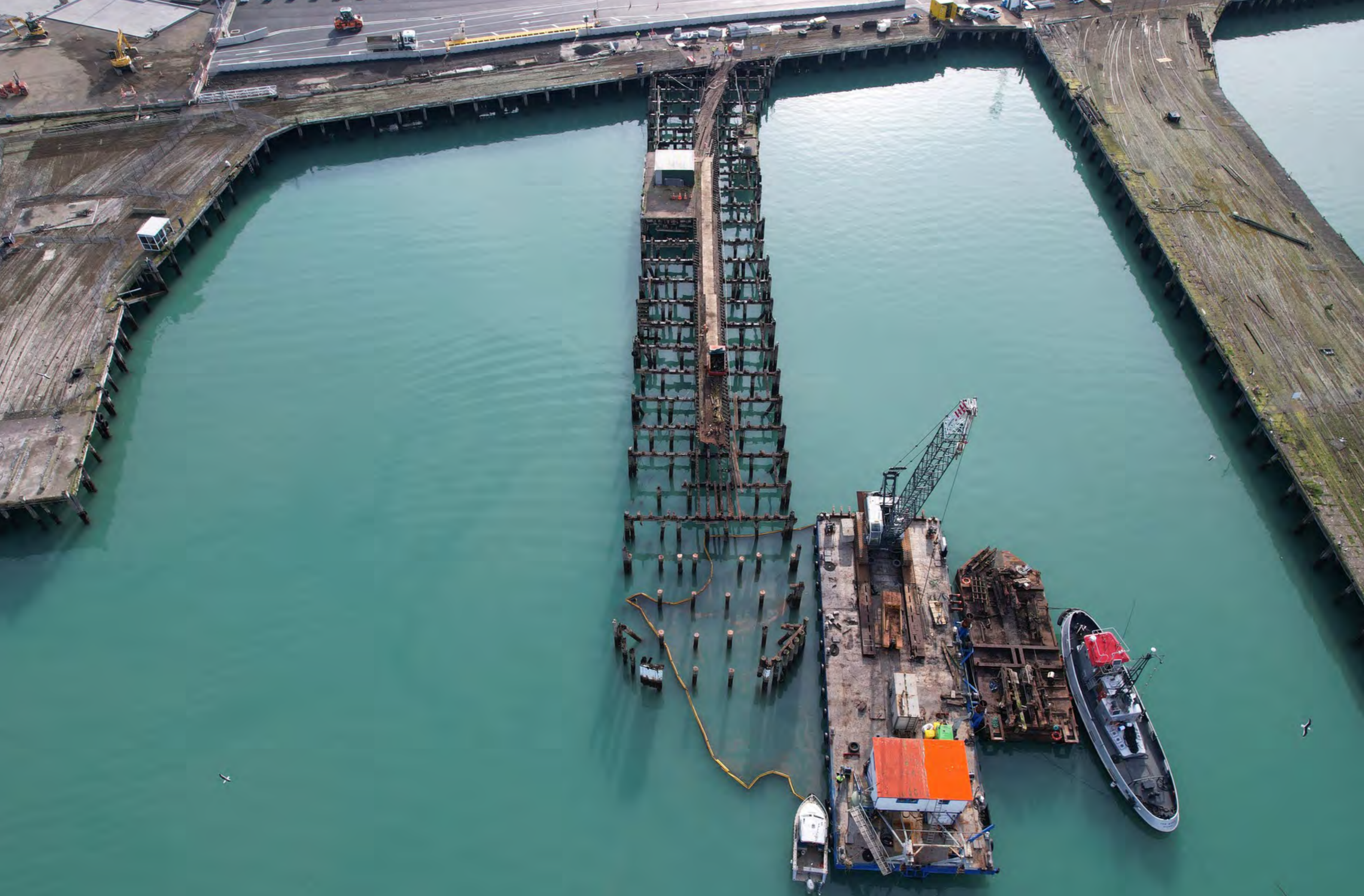
ALANA FROM SMITH CRANE AND CONSTRUCTION, AT LYTTLETON PORT, CHRISTCHURCH - SMITH CRANE AND CONSTRUCTION'S CIVIL TEAM HITS THE WATER TO DISASSEMBLE JETTY
