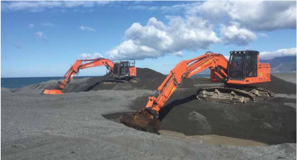
Draining the water from Lake Onoke out to the ocean – JPS Earthmoving.
