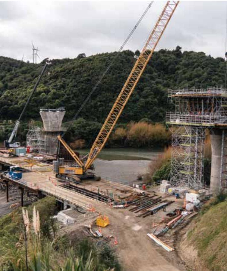
Work on the three concrete piers for the 300 metre long Parahaki Bridge over the Manawatū River
