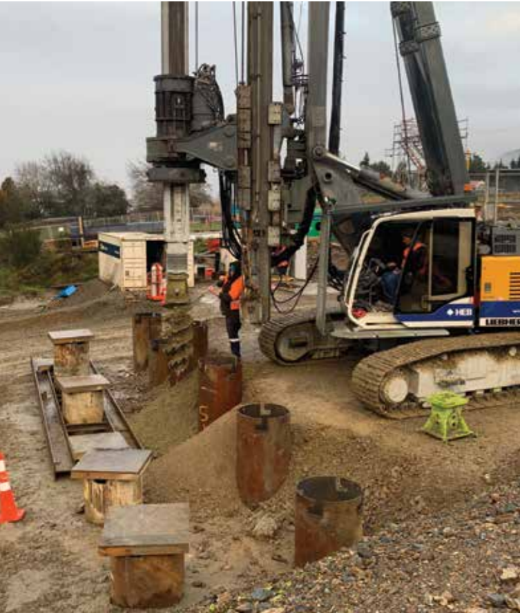
Drilling pile foundations for an abutment for the Clutha River bridge at Beaumont – HEB Construction
