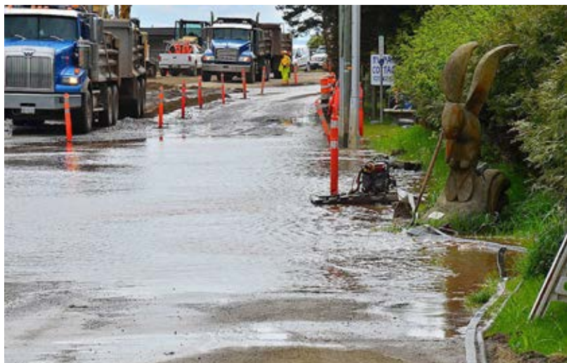
Water can pool in various places, especially in construction environments where the topography has changed. This photo is an extreme version, but even a blocked drain due to construction debris can have an impact on the safety of vulnerable road users in a worksite. Image Credit Ixviii: Campbell River Mirror.
