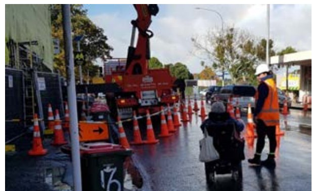
Having staff on hand to escort and assist those with disabilities is a very effective way to ensure sites are able to be navigated safely by even the most disadvantaged of users. Image Credit lxxxi: Parallax.
