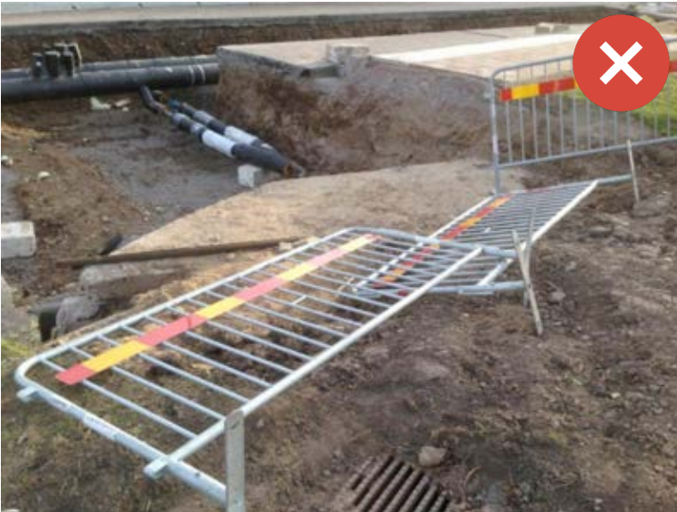
Fences to prevent access to hazards but have fallen over, creating risk for vulnerable road users. Image Credit Ivi: Sweden National Road and Transport Research Institute 44 .
