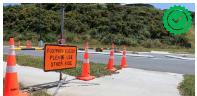
Example of footpath closure (using other side) utilising an existing pedestrian refuge. Image Credit xlix: Danny Wood.
