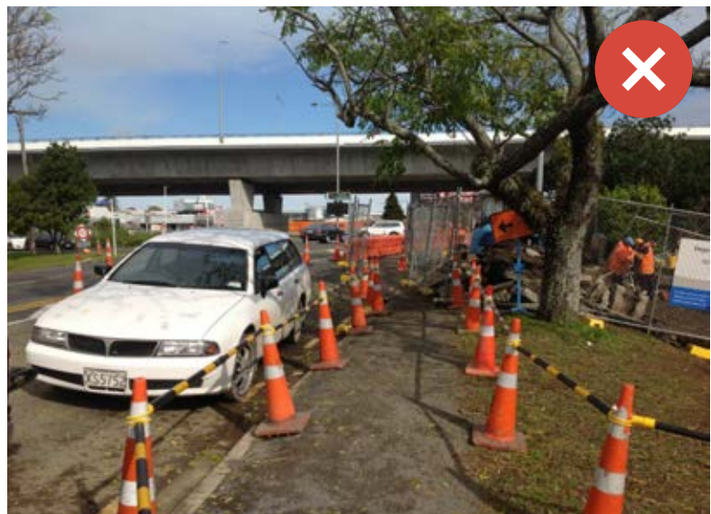
Temporary walkways should be safe, obvious, and smooth and stable. In this case the path narrows considerably, the sign is obscured, there is an unsafe kerb drop off, and many trip hazards. Image Credit cviii: Parallaxx.
