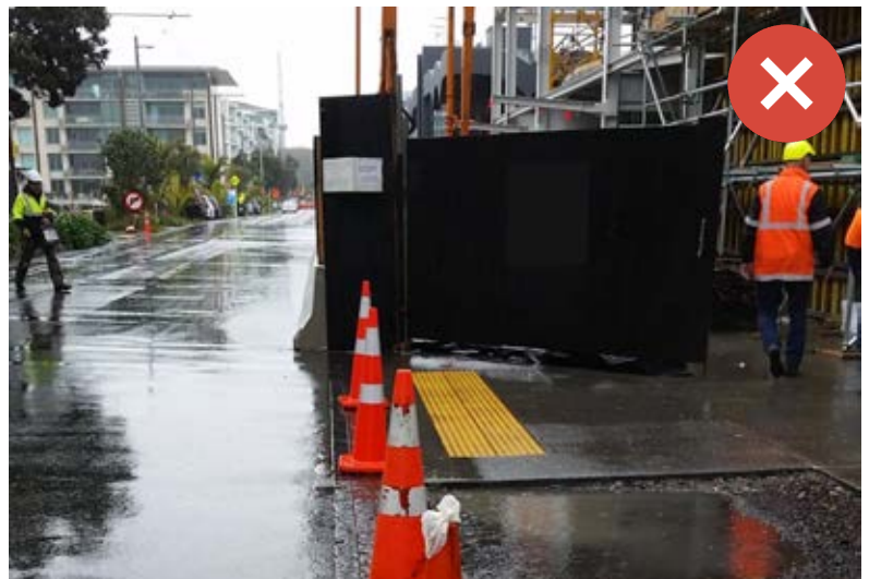
This crossing point is significantly compromised by the site hoarding, meaning anyone crossing from right to left (as viewed) would have no visibility of oncoming traffic. Image Credit lxvii: Parallax.
