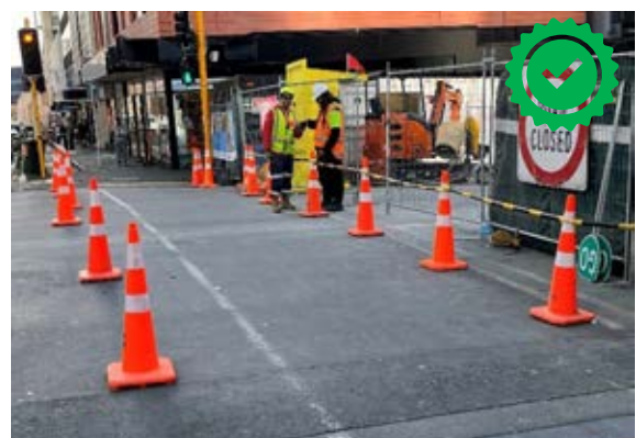
Existing pedestrian crossing maintained with full width and enhanced by some adjacent cones for clarity. Image Credit xli: Betty Mitrova.
