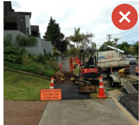
Cone Bars do not stop users and provide little security that access to hazards is prevented. In this instance its clear a user can bypass the control measures into the hazard. Image Credit Ixxvi: Parallax.
