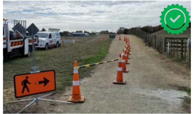
This example shows a narrowed existing path with a method to prevent access to the hazard area and directional signage. One improvement would be ensuring the method preventing access is particularly clear at the entry points (closest to the camera) to make sure pedestrians can't get through, especially at the point of the change in their direction. Image Credit xliii: Traffic Management Hawkes Bay.
