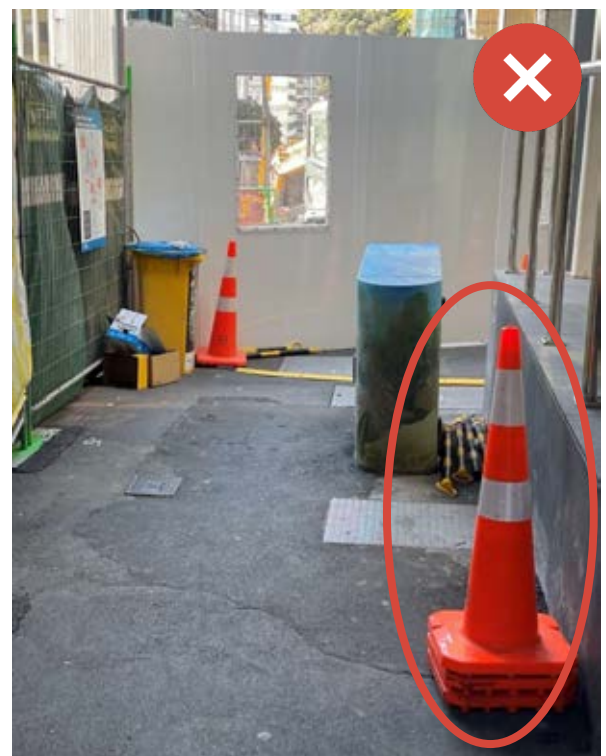
Equipment left in or adjacent to pedestrian routes that is unused only serves to add obstacles or hazards to users. Image Credit Ivi: Betty Mitrova.
