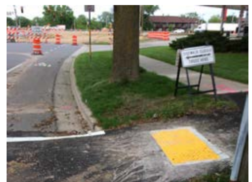
Tactile Ground Surface Indicators are an important measure for the safety of pedestrians, even at temporary crossing points. They should be considered in accordance with best local practice. Image Credit c: UW-TOPS Lab.
