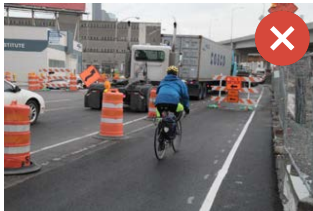
Cyclist detour with no clear safe arrangement with the nearest traffic lane at the point of detour. Image Credit li: Washington State Department of Transportation.
