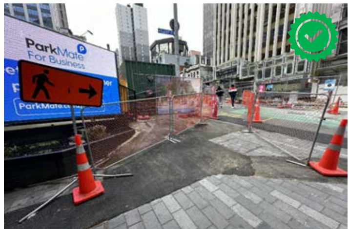
An example of a temporary diverted pedestrian route into a closed road space. One improvement is a few trip hazards that are visible. Image Credit xlv: Parallax.
