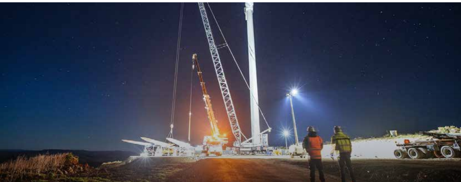
Alana from Smith Crane and Construction, at Kaiwera Downs WindFarm, Gore - Our Windfarm team installing a turbine early in the very early hours of the morning.
