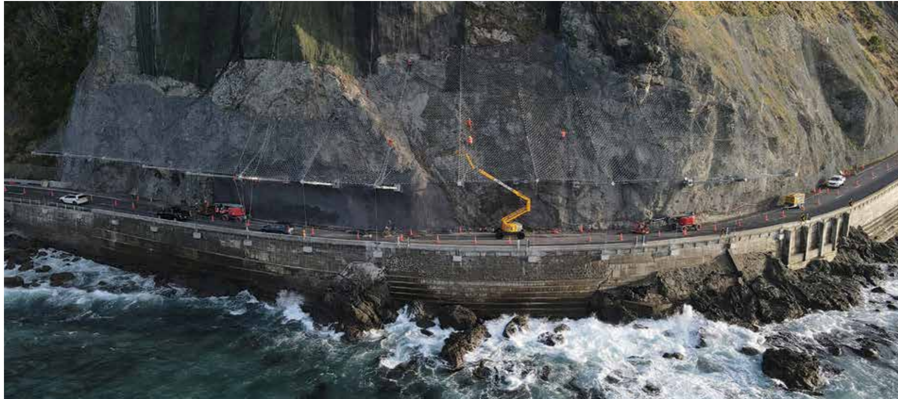
Kaikoura rockfall protection.
