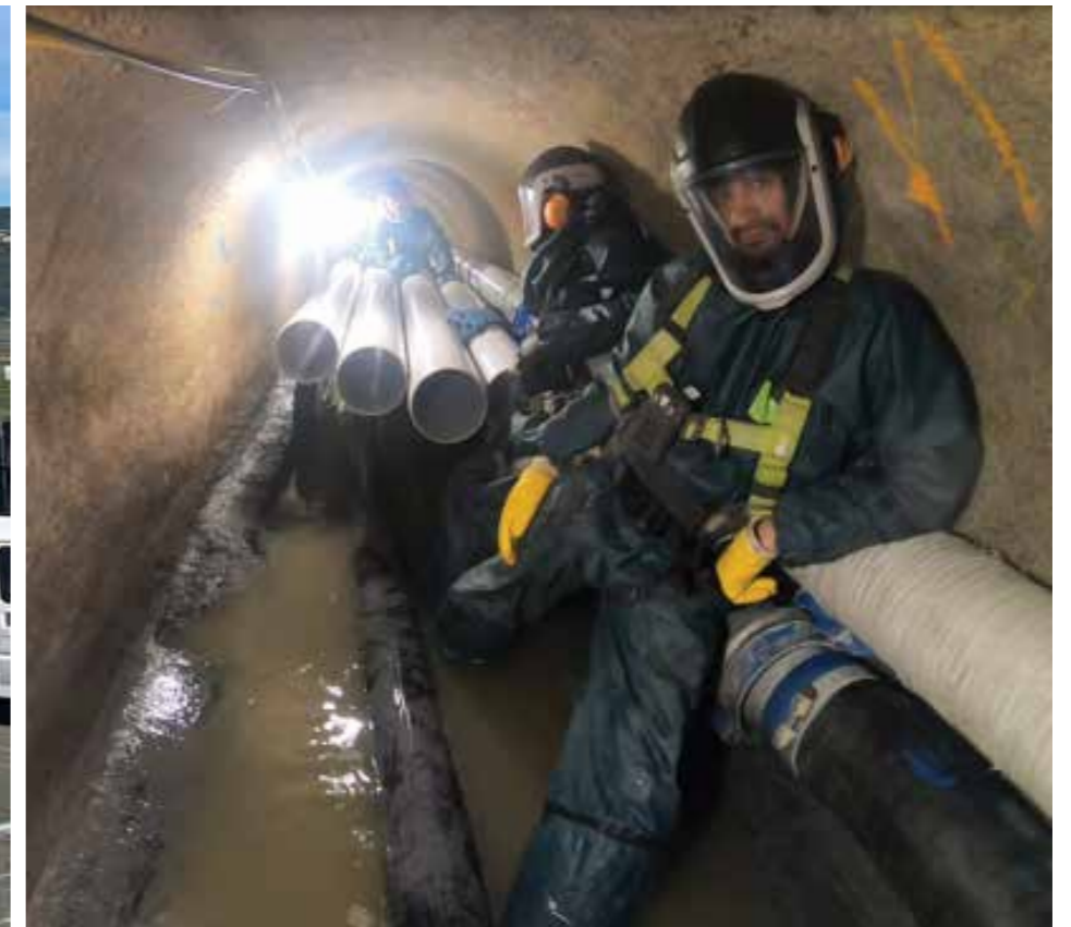
Brian Perry Civil team working on the Mount Albert Sludge Pipeline repairs.
