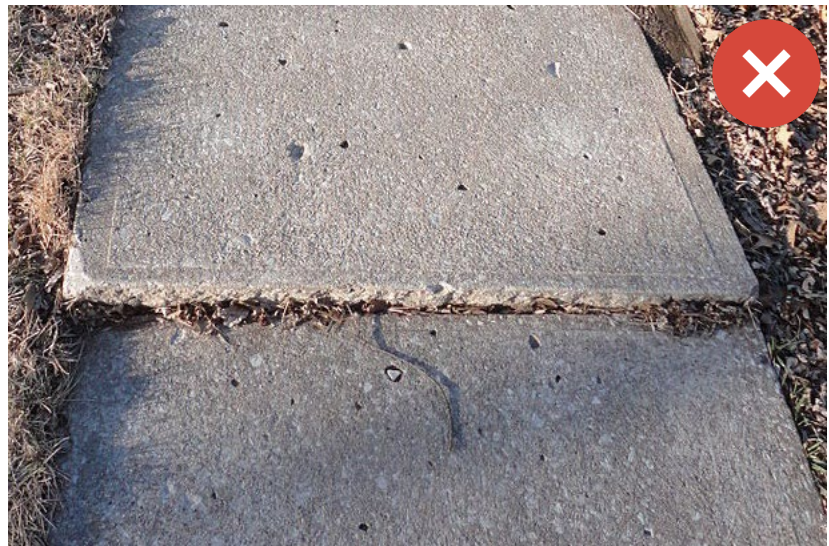
Any footpath (temporary or not) has risk of trips where there are level differences in the surface. Any step thicker than a pencil is a potential trip hazard and should be addressed by fixing the path (preferred), and if not reasonably practicable, delineating and marking the hazard so it is clearly visible. Image Credit cvi: Wikimedia Commons.
