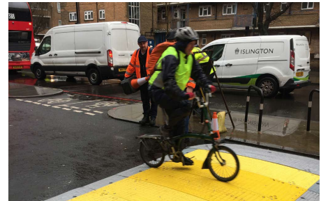
Some excavation covers are rated for vehicle and VRU use. Image Credit lxxxiii: Transport for London.
