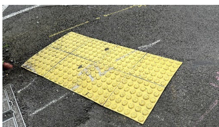
Tactile ground surface indicators can be installed easily and quickly. Image Credit xcix: Parallax
