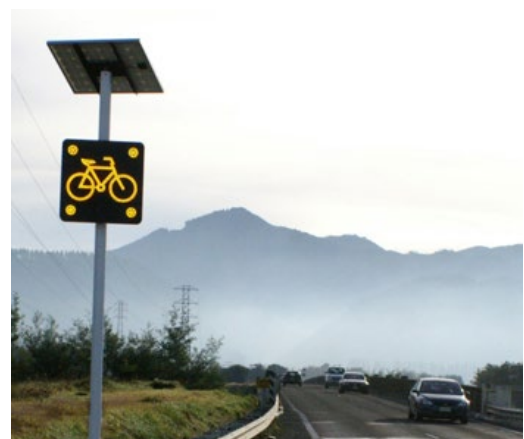
Electronic responsive signage can enhance the safety of VRUs. There are temporary options available for use in TTM environments. Image Credit Ixxiii: HMI Technologies New Zealand.
