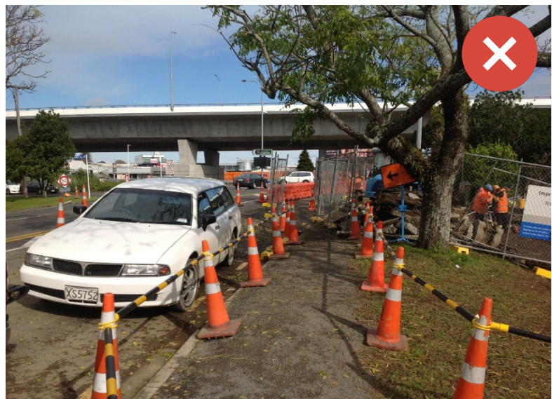
Temporary walkways should be safe, obvious, and smooth and stable. In this case the path narrows considerably, the sign is obscured, there is an unsafe kerb drop off, and many trip hazards. Image Credit cviii: Parallaxx.
