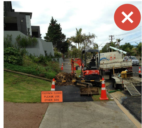
Cone Bars do not stop users and provide little security that access to hazards is prevented. In this instance its clear a user can bypass the control measures into the hazard. Image Credit Ixxvi: Parallaxx.
