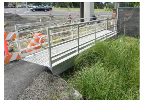
Temporary bridges should be stable and embedded into the pathways either side so there are no trip hazards for users at either end. Image Credit cxiv: Oregon Department of Transport.
